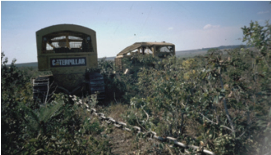
Figure 2.6 A much used method for deforestation: dragging a long metal chain between two bulldozers. © Ulrike Bickel
